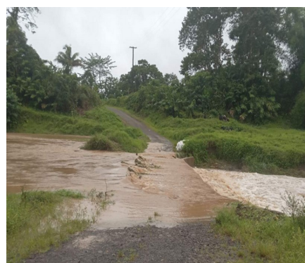
Figure 12f: Vatulili Crossing on the 13 th . Source: Fiji Roads Authority.
