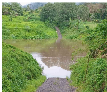
Figure 12i: Wairua crossing on the 30 th . Source: Fiji Roads Authority
